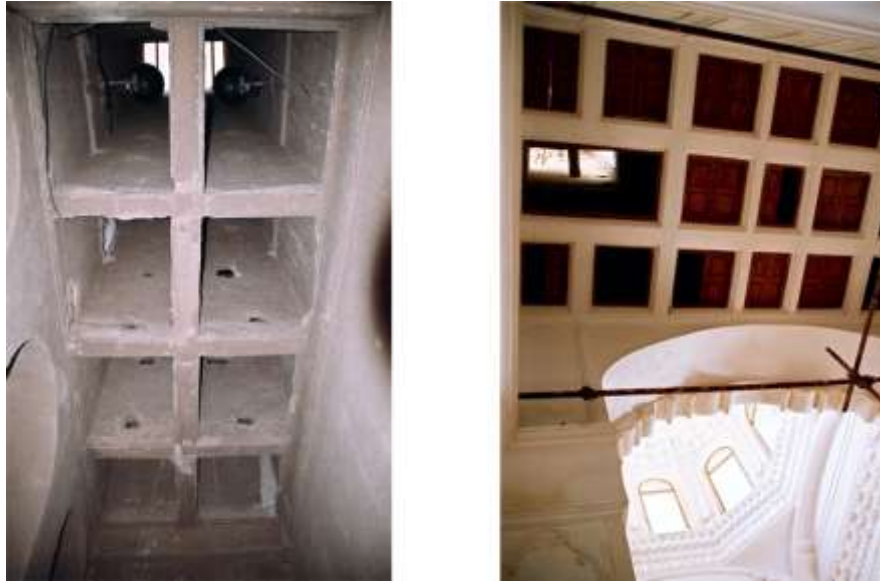
Figure 8: The view of wind catchers from the bottom of the chamber (Zandi, 2006)
