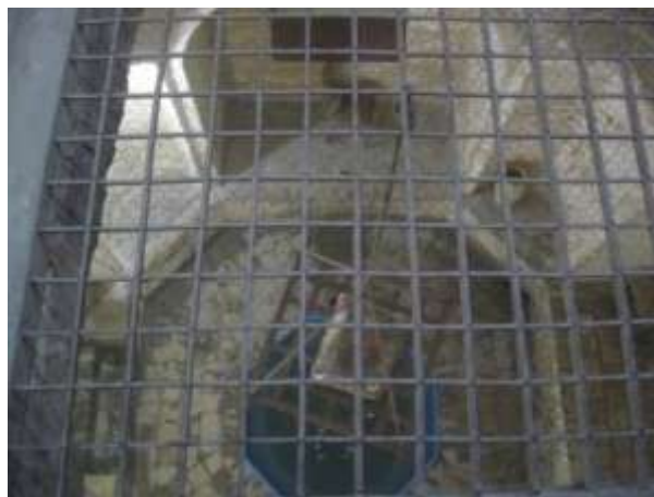
Figure 42: Hole in the ceiling of basement spaces in Yazd traditional houses
