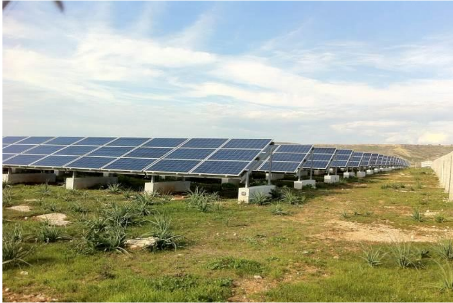
Figure5.5: Photograph of the PV plant 20 km 2 land, looking south-west.
