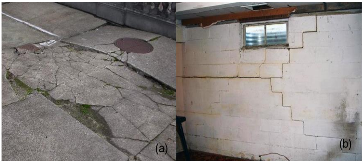
Figure 2.1: Cracks in (a) pavements and (b) buildings
