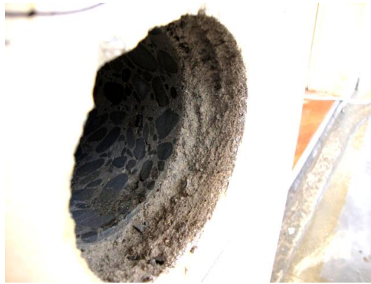
Figure 4.24: showing drilled area after taking the sample from column
