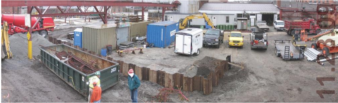
Figure 20: Steel Yard Remediation Project in progress 2009 (Source: Steel Yard Flickr Photo Stream, http://www.flickr.com/photos/thesteelyard )
