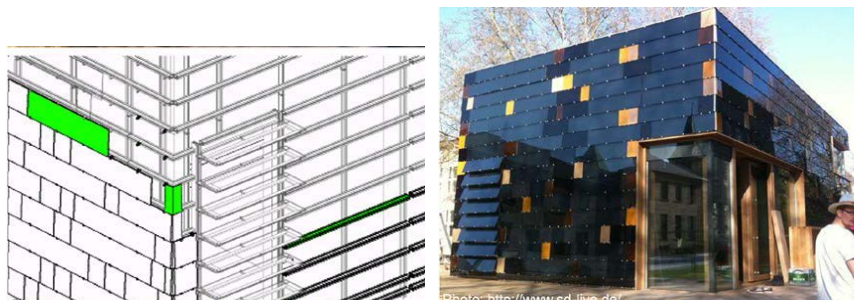
Figure 1.25 (left): Integration of PV Shingles on the Façade of Surplus-home of Team Germany, (Right): Jointing of PV Shingles used, Jointing in the Multifamily Dwelling
