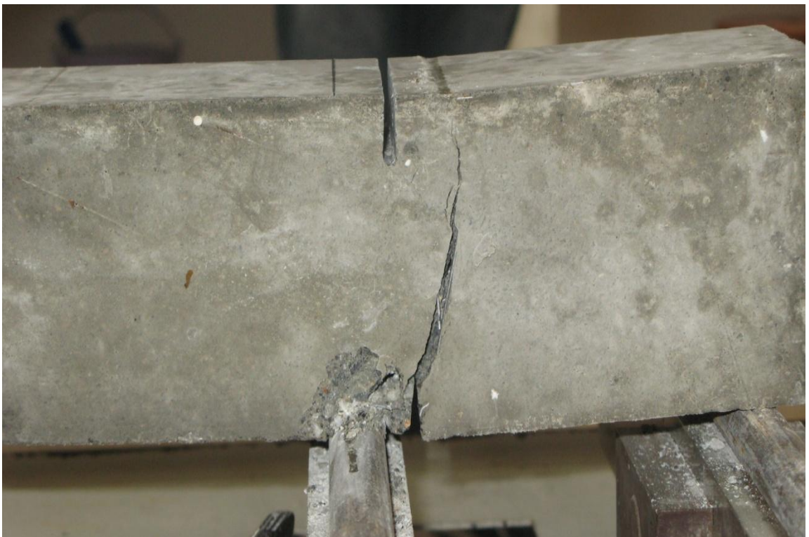
Figure 65: moment of shear cracking
