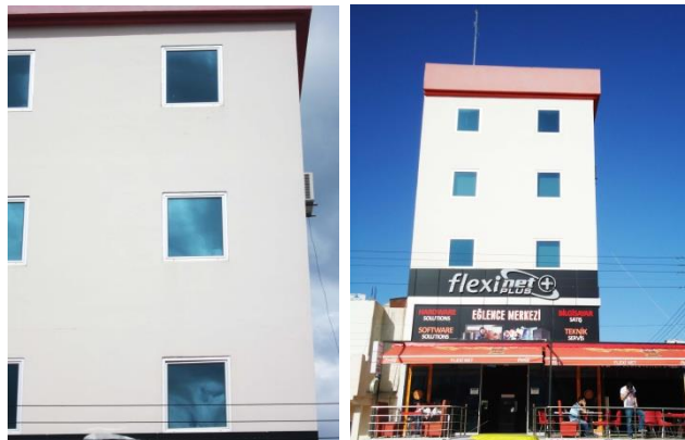
Figure 3.21: This Building Has No Shading Devices in All Facades (Photos taken by author)
