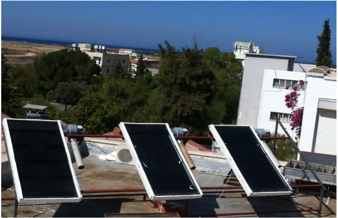
Figure A1: Solar air heater collectors.
