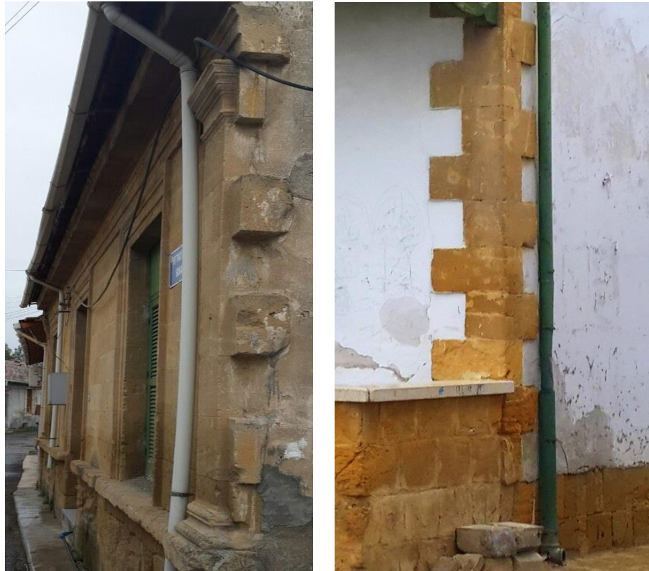
Figure 41: Exposed Bond Stone at the Corner
