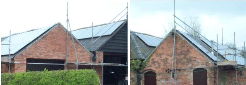
Figure 3.141: General View of the Panels Installed on the Two Pitched Roofs
