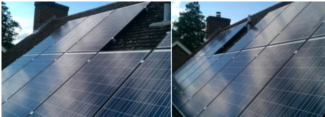
Figure 3.138: Poly-crystalline Panels were Installed on the Roof and Organized Portrait
