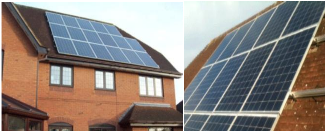
Figure 3.136: General View of Poly-crystalline Panels Located on the Roof Surface (Portrait Organization)
