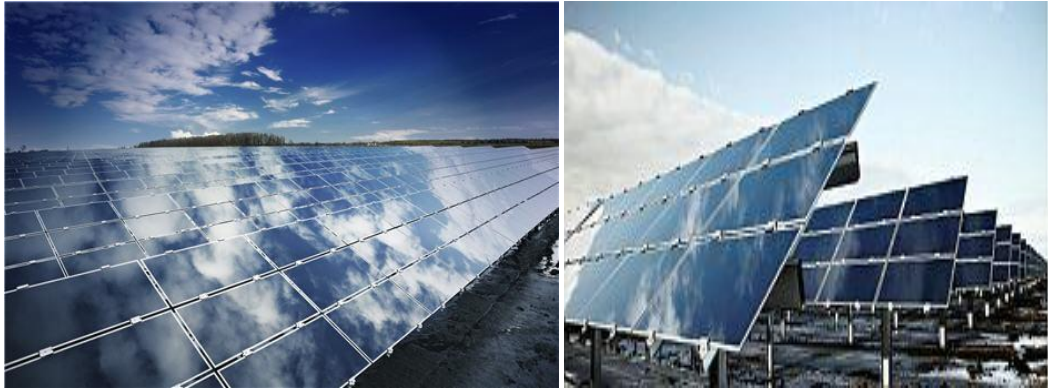
Figure 3.91: Different Views are taken from Photovoltaic Power Plant (Enbridge, 2010)
