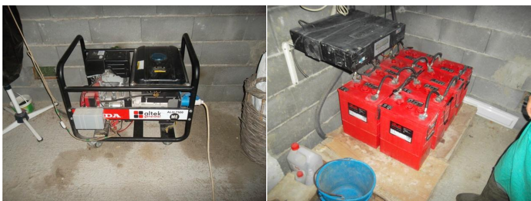
Figure 3.63: Photo shows Generator and 8 Watery (Juicy) Batteries (Taken by author)
