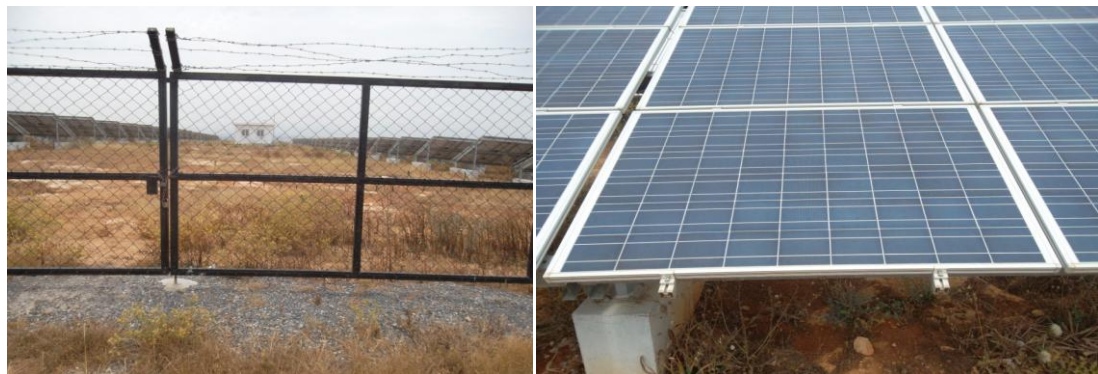
Figure 3.45: Photo shows the Outside View and Panel Cell Type (Taken by author)
