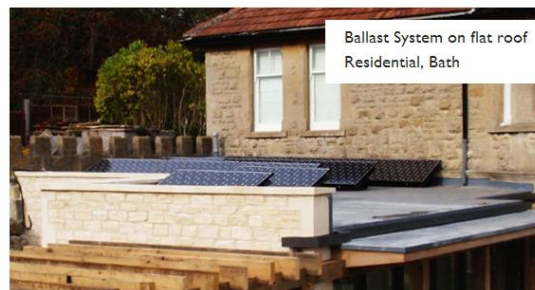
Figure 2.17: Photo shows the Flat Roof PV Application Supported with Plastic Tubs (Horizon Renewables, 2013)
