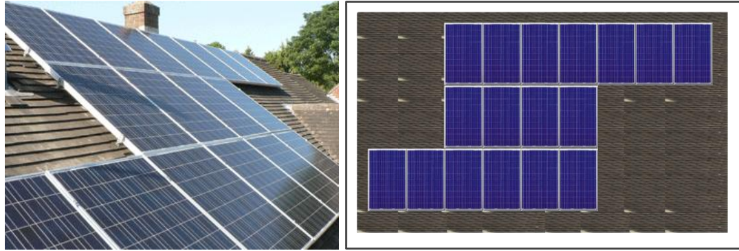
Figure 3.128: Photo shows the 5 th House Panel and the Top View (Portrait Organization)
