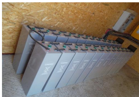
Figure 3.15: Photo show 24 Numbers of Batteries (Taken by author)
