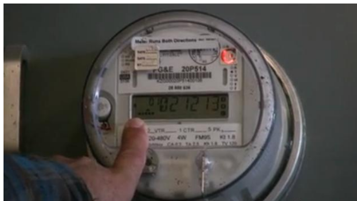
Figure 3.85: Photo shows the Electric Meter (Youtube, 2013)
