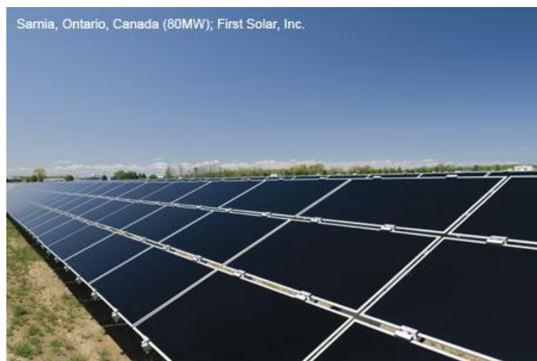
Figure 3.93: Thin-film Modules were mounted to the Profile Carriers (SolarServer, 2010)
