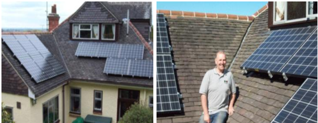
Figure 3.130: Photo shows the General View of the Panels
