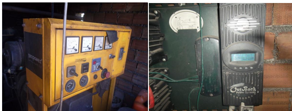
Figure 3.71: Photo show Generator, Mate Control and Charge controller (Taken by author)
