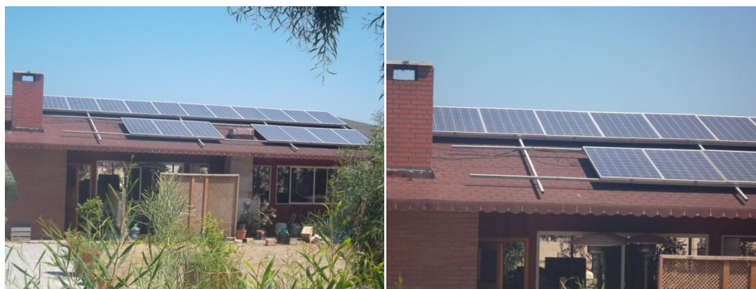
Figure 3.68: General View of the Panels Added on the Pitched Roof (Taken by author)
