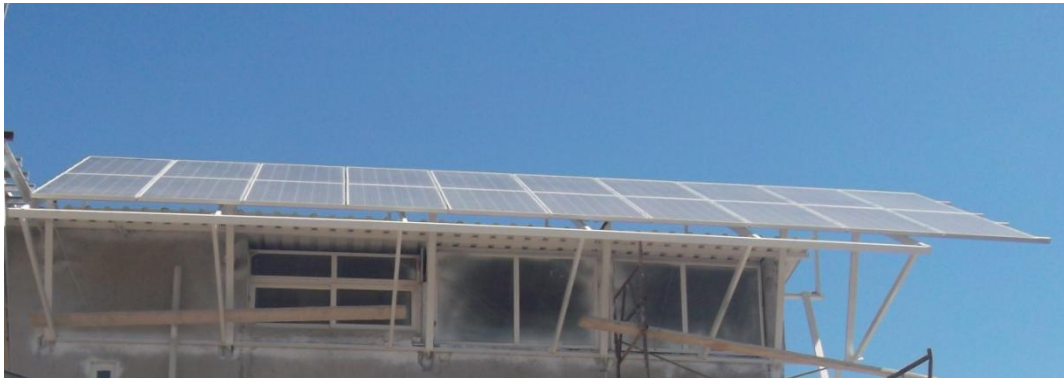
Figure 3.76: 20 Panels Organized Portrait added on the Roof (Taken by author)
