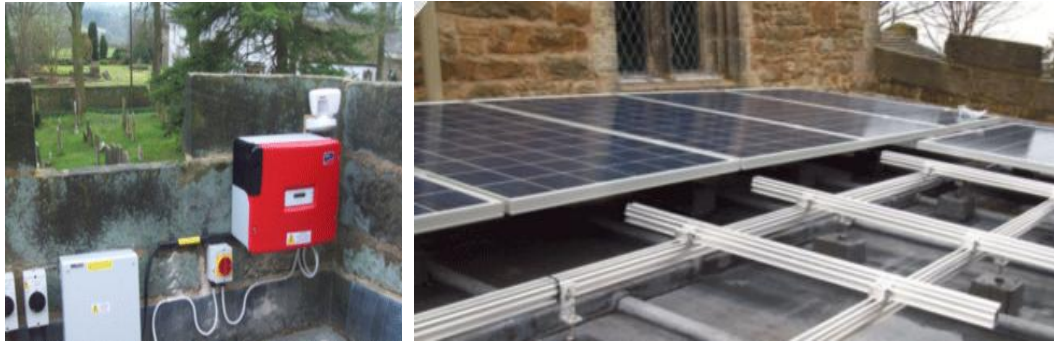
Figure 3.147: Photos are showing inverter and the structure of the profile carriers
