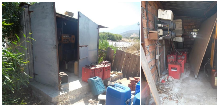
Figure 3.70: Photos show Batteries (Taken by author)
