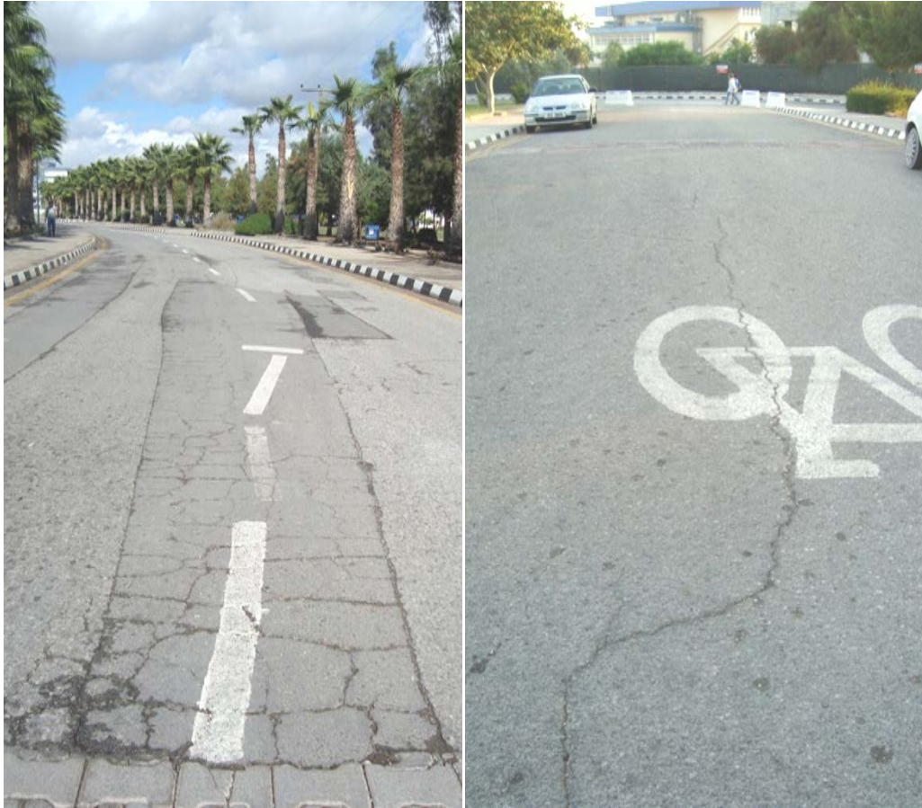
Figure 4.14: Patching (sect. SP 03).Figure 4.15: Longitudinal Cracking (sect.ACA 20).
