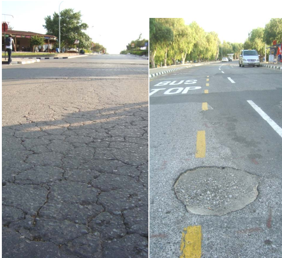
Figure 4.8: Alligator Cracking. (sect. ACA 01).Figure 4.9: Pothole (sect. DOR02).
