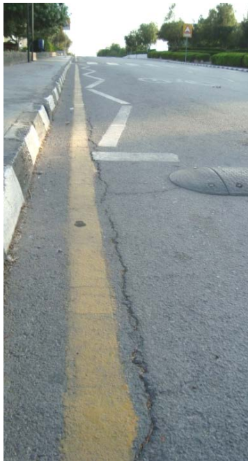
Figure 4.12: Edge Cracking (sect. ACA 02).
