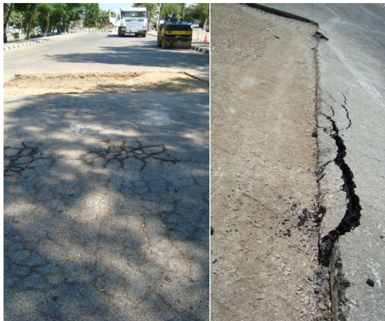
Figure 1.2: Alligator cracks not maintained. Figure 1.3: Cutting deteriorated area.
