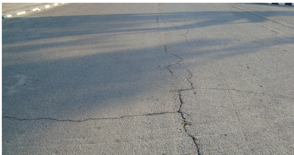
Figure 4.10: Block Cracking (sect.ACA 16).
