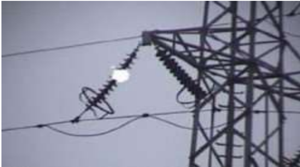
Figure.2.2: Corona effect on power lines [7]
