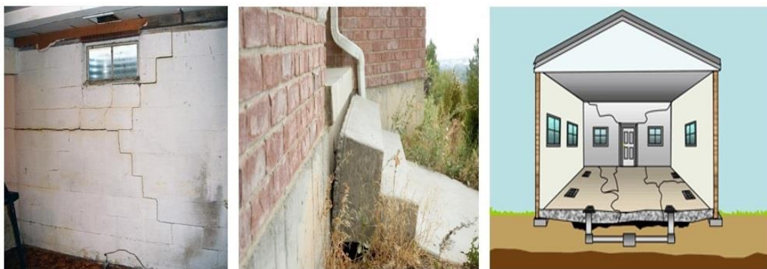
Figure 2.2: Damage of expansive soils on structure
