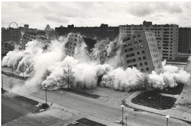
Figure 2.9. Explosion of Pruitt-Igoe ( www.heathershimmin.com ).
