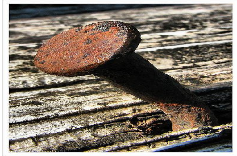
Figure 10. Rust on metal surfaces [11]
