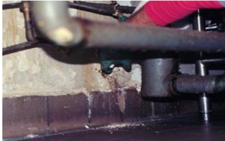
Figure 5. Standing water in ducts [7]
