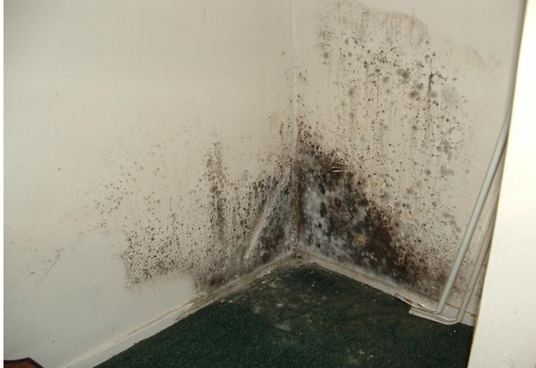
Figure 12. Mold on ceiling, wall and material [64]
