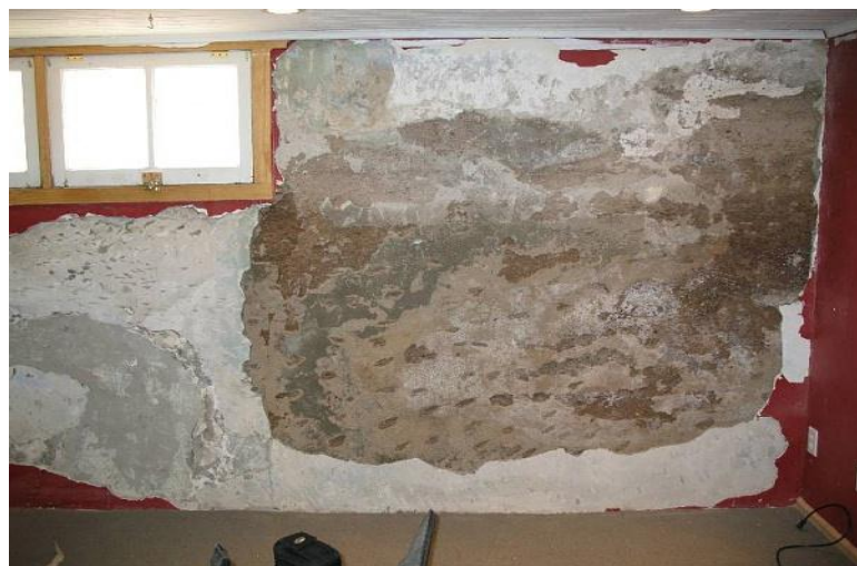
Figure 2. Softening of wall surfacing material [2]
