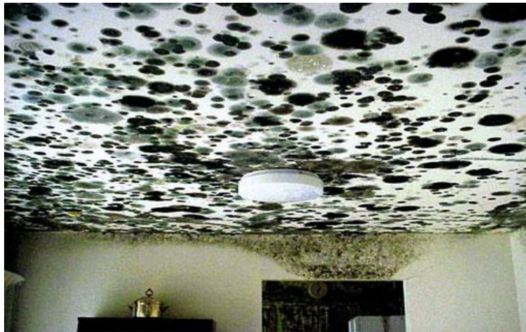
Figure 11. Mold on ceiling, wall and material [64]
