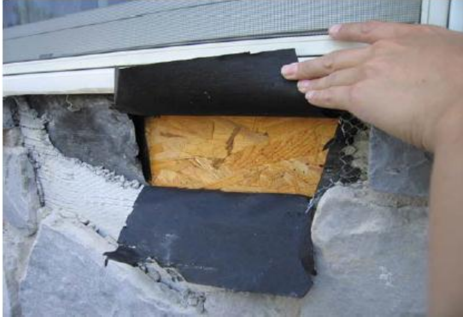
Figure 32. Measure the moisture content inside the wall the stone and cladding are removed for installing the probe type moisture meter. [51]
