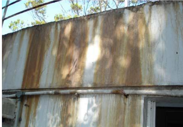
Figure 8. Discoloration of materials [9]
