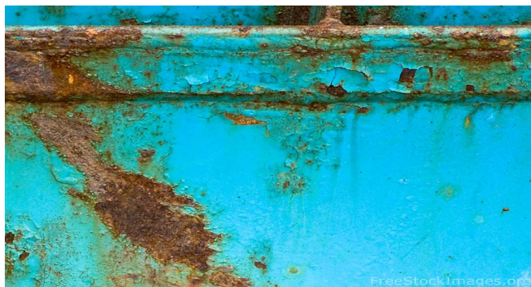
Figure 9. Rust on metal surfaces [10]
