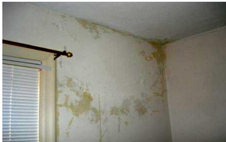
Figure 7. Discoloration of materials [65]
