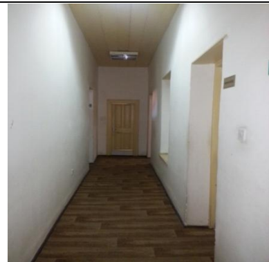
View showing the interior of first floor with carpet used to cover the original wooden floor
