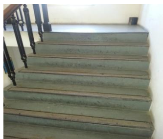
Cemented stair case area leading to the second floor from first floor
