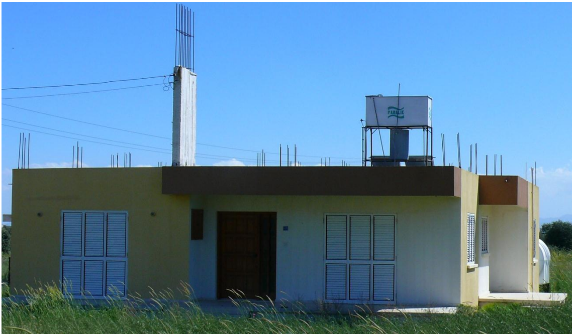
Figure 1.1: A building appears to be incomplete, due to the starter bars left on the roof
