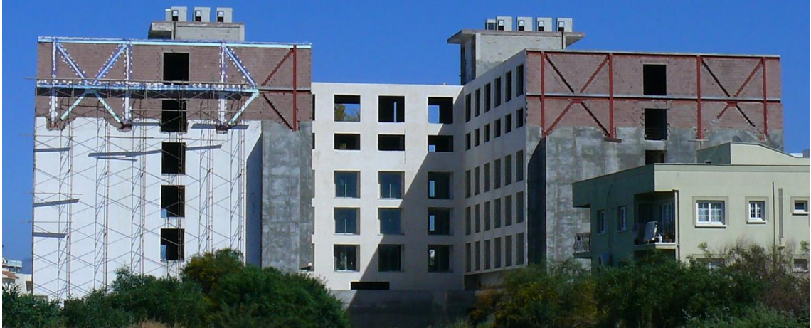
Figure 1.2: One of the application; first four stories made of reinforced concrete and upper two stories made of structural steel.
