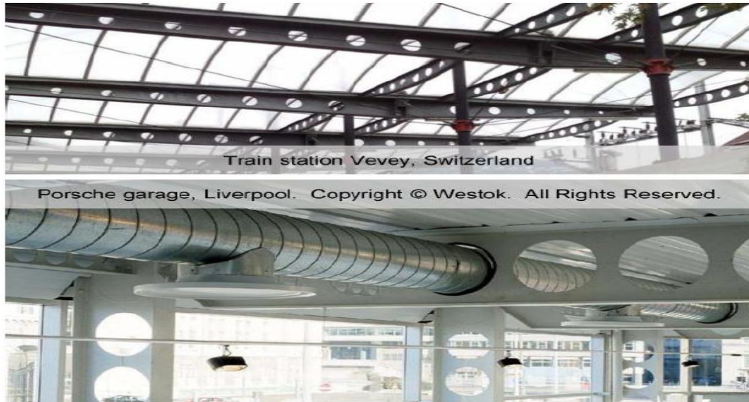
Figure 6 Cellular beams facilitating the passage of services (Westok, 2013)
