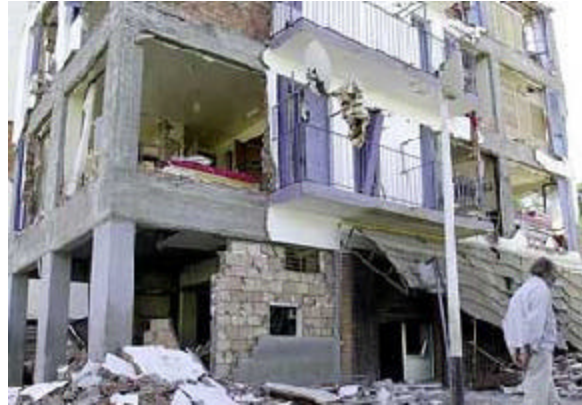
Figure 5.6: A reinforced concrete structure affected by 2003 Earthquake in Algeria (Carrillo and George, 2004).
