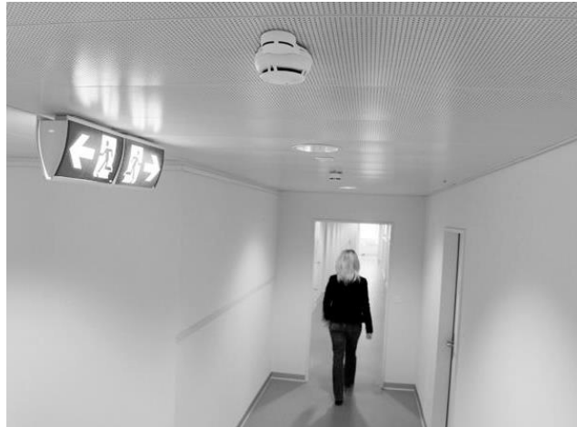
Figure 3.47: emergency exit sign and fire detector (Siemens, 2013)
