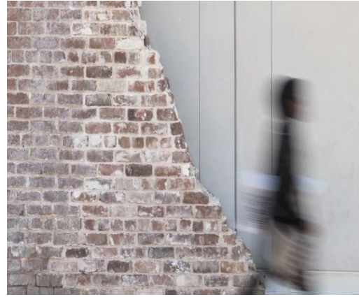
Figure 4.71: Vicinity of New and Old Material in the Museum Structure (SCAD Museum of Art Featured Artists, 2013)
