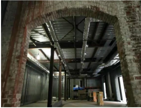
Figure 4.70: ventilation system beneath the ceiling, SCAD Museum of Art (SCAD museum of art, n.d)
