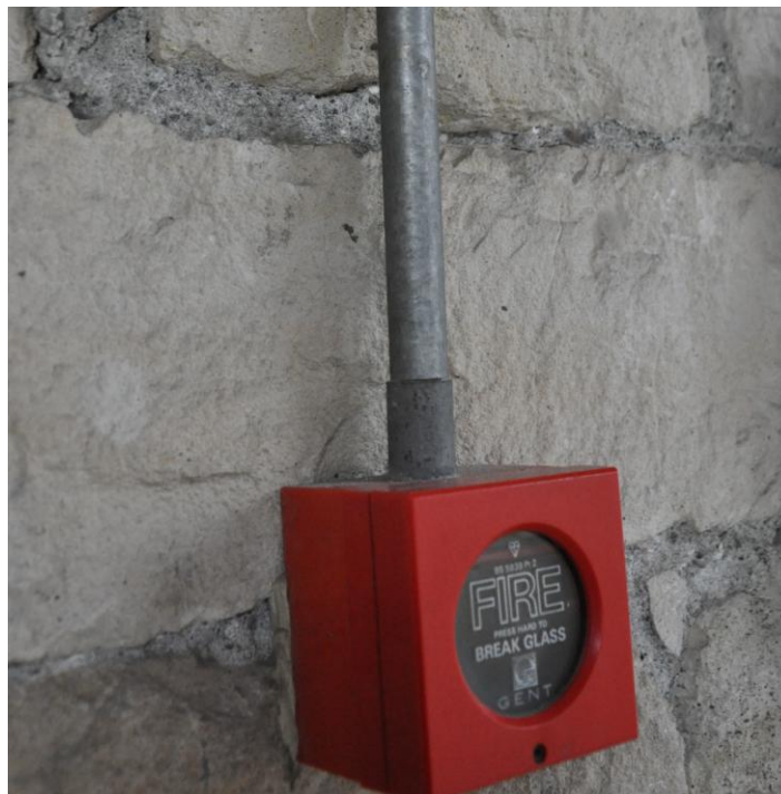
Figure 2.34: Fire Security System (Türker Archive, 2010) Minimum Intervention has been achieved in the additional Systems.
