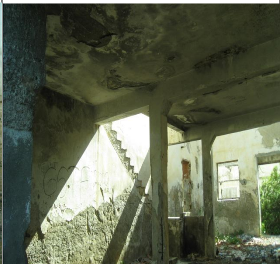
Figure 4.20: Demolished Double Storey Part of Zeyko Olive Oil Factory, Kyrenia (Golmakani archive, 2009)
