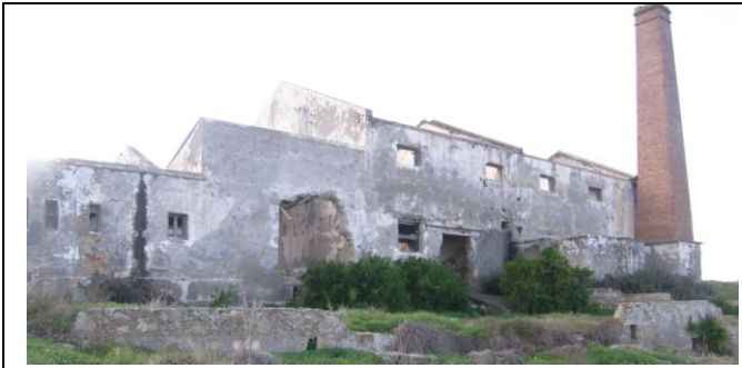
Figure 4.21: Deteriorated South-East Façade of the Zeyko Olive Oil Factory, Kyrenia (-Golamakani archive, 2009)
