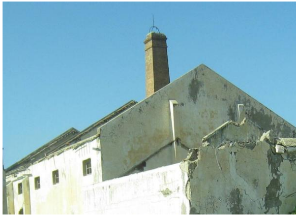
Figure 4.25: Slopy Deteriorated Roof of Zeyko Olive Oil Factory, Kyrenia (Golmakani archive, 2009)
