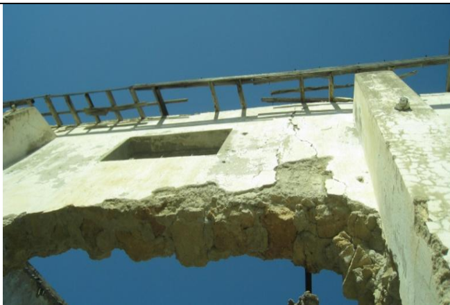
Figure 4.23: Deteriorated Mud Brick Load-Bearing Wall of the Zeyko Olive Oil Factory, Kyrenia (Golmakani archive, 2009)
