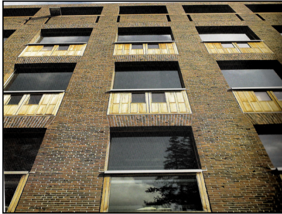
Figure 4.30: The façade of the Exeter Library, showing the decreasing the brick exterior columns as they rise, reflecting their diminishing structural loads.
