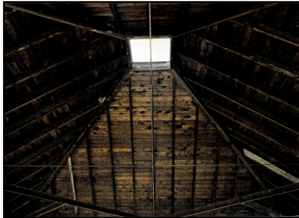
Figure 4.2: Bathhouse's roof, showing Rafter, wood beam, secondary beam and cables (McCarter, 2005, p.98)
