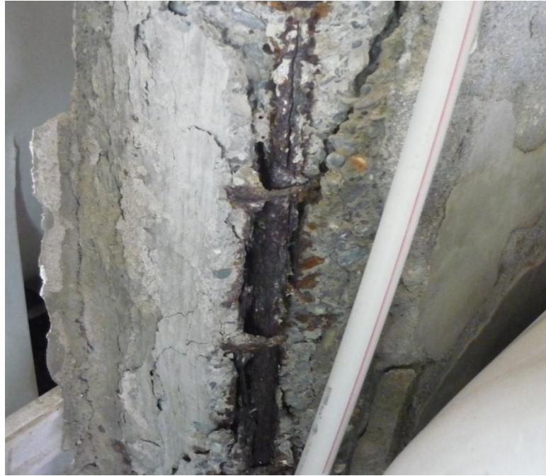
Figure 6.1: High Corrosion Levels in Columns
