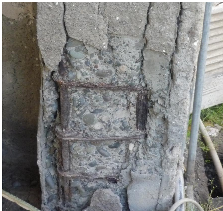
Figure 6.2: Extinction of Concrete Cover Due to High Levels of Corrosion
