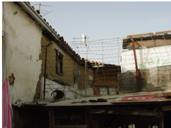
Figure 6: Current condition of rear part of the dwellings.
