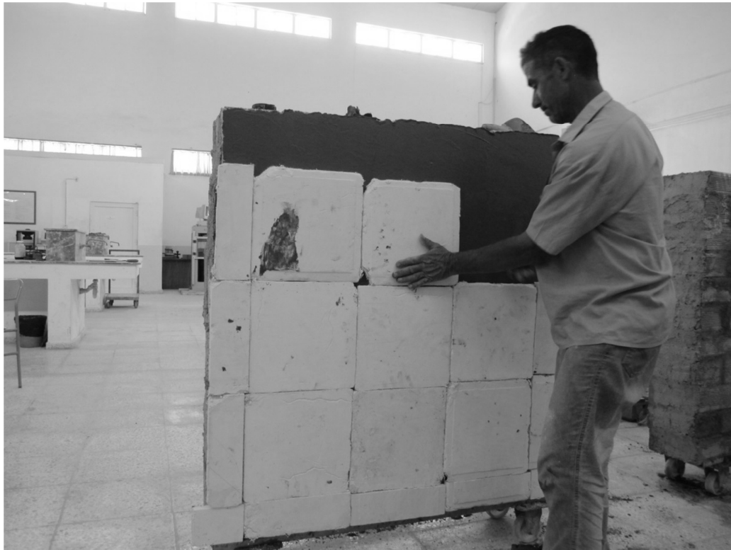
Figure 3.22: The Samples Attached to the Wall Type II with 1 mm Tile Glue
