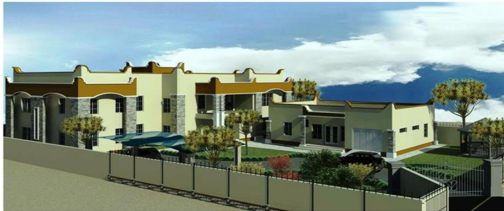
Figure 4.13: Shows postmodern residential building under construction interplayed with many color. (Photo by author)
