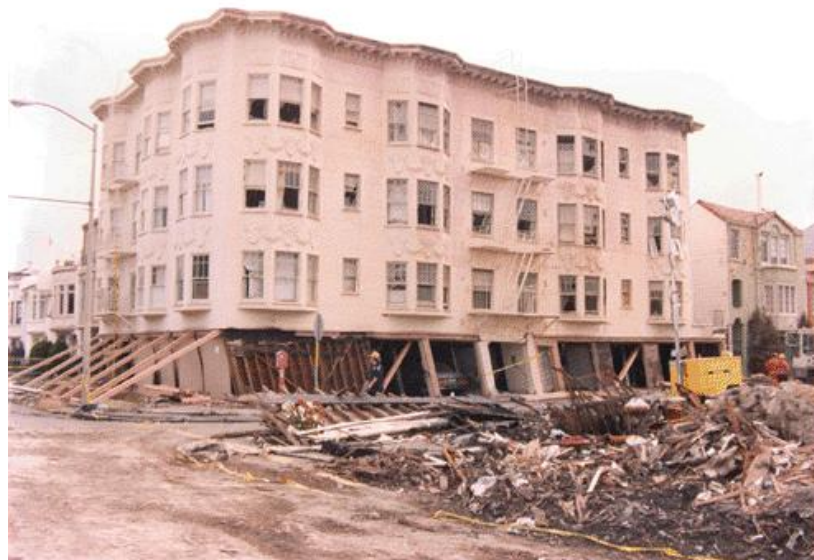
Figure 3.19. Collapse due to Soft or Weak Storey (Tolleson, 2010)
