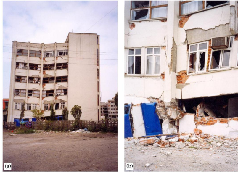
Figure 3.5. A Building Damaged due to Torsion Eccentricity (Özmen and İ.Ünay, 2007)
