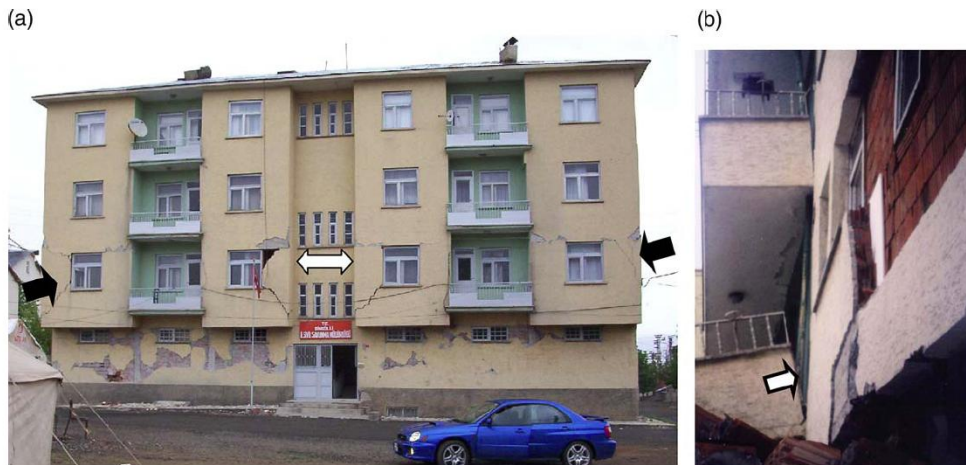
Figure 3.34. Heavy Cantilevers and Balconies (Doğangün, 2004)
