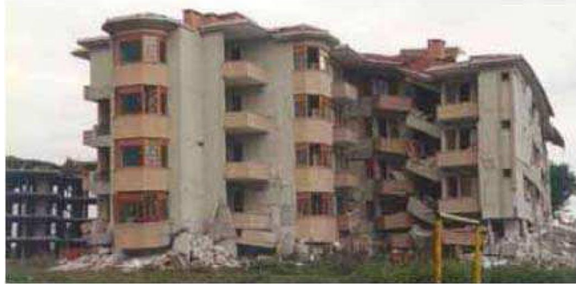
Figure 3.12. Illustration of a Building that was Ruined after Marmara Earthquake, Attributed to Irregularities in Plan (Balyemez and Berköz, 2005)
