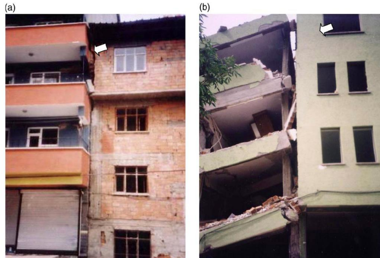
Figure 3.27. Hammering Effect for Adjacent Building (Doğangün, 2004)
