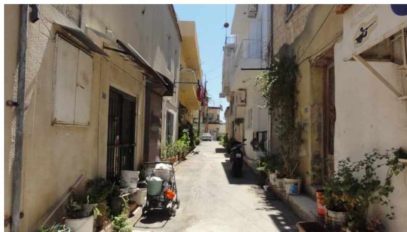
Figure 28: Condition of Buildings
