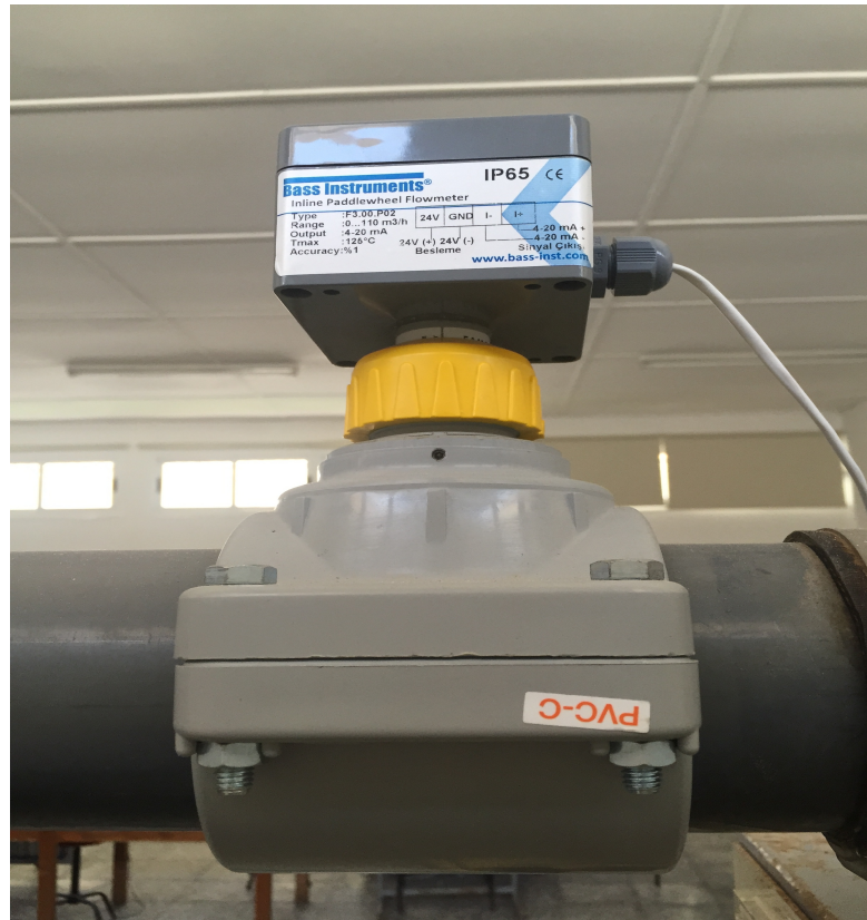
Figure 3.20: Installed Paddlewheel flow sensor
