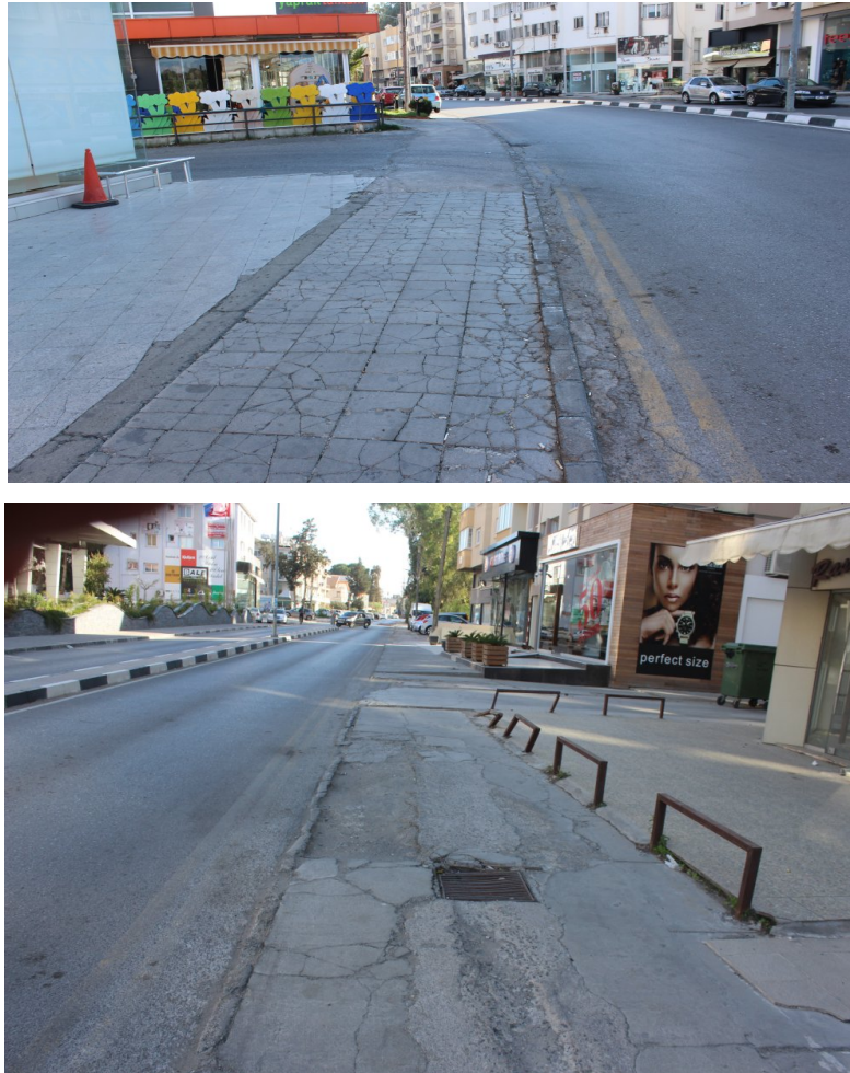
Figure 3.23. Damaged Flooring and Unattended Pavement
