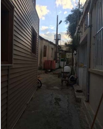
Figure 44: Inappropriate maintenance on facades
