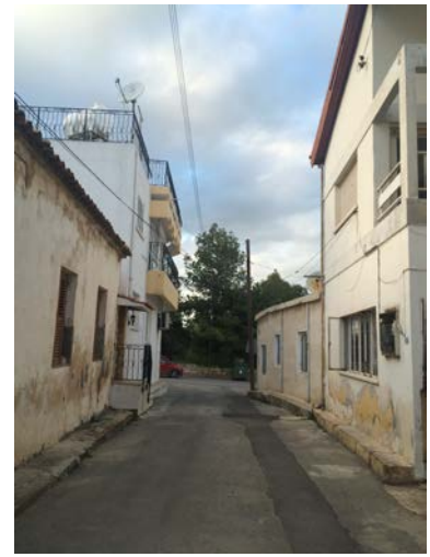
Figure 49: Detoriation on facades
