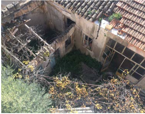
Figure 20: Deteriorated building in Berhan Pasha Street
