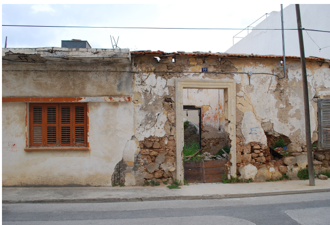
Figure 2.1: An abandoned house in the Walled City of Famagusta, (Author, 2013)
