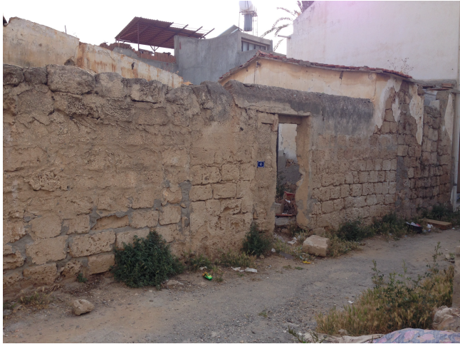
Figure 2.4: Deteriorated façade condition in the Walled City of Famagusta, (Author, 2013)
