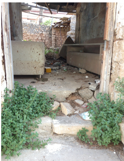
Figure 4.21: An abandon house without door and trash inside (Author, 2013)
