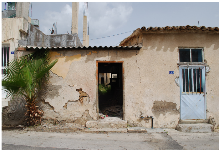
Figure 4.20: An abandon house with no door, broken window, deteriorated façade and structure and trash inside (Author, 2013)
