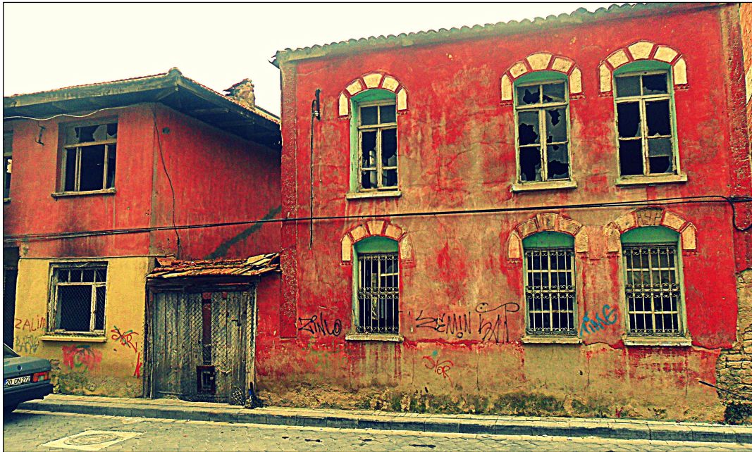
Figure 2.5: Physical disorder (poor façade condition, broken windows and graffiti), URL.3
