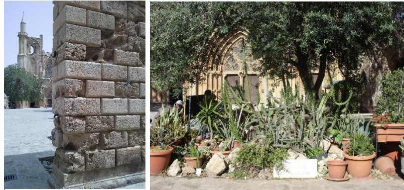
(c) Erosion of Venetian Palace's walls (d) Lack of proper landscape design
