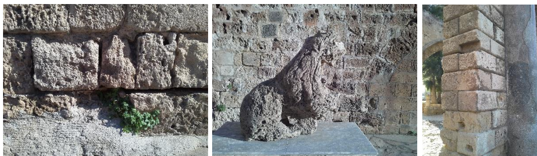
(a) Erosion of historical buildings' facades (b) Lion statue of the Sea Gate (c) Walls of Venetian Palace
