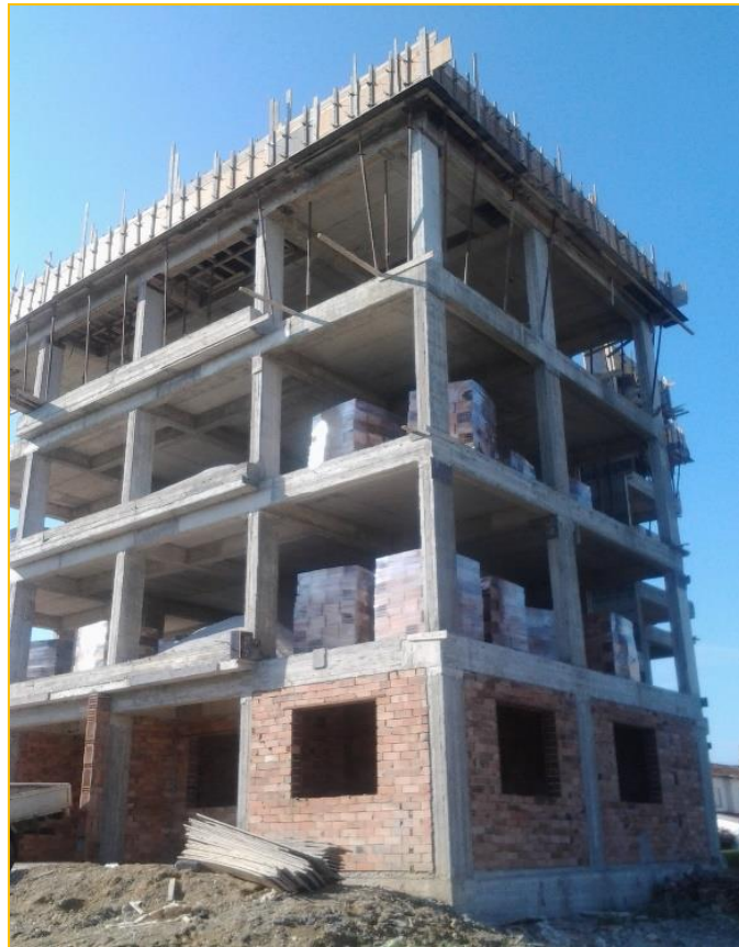
Figure 14. The building number 3 East side (Photo taken by author in 27th of December, 2014)
