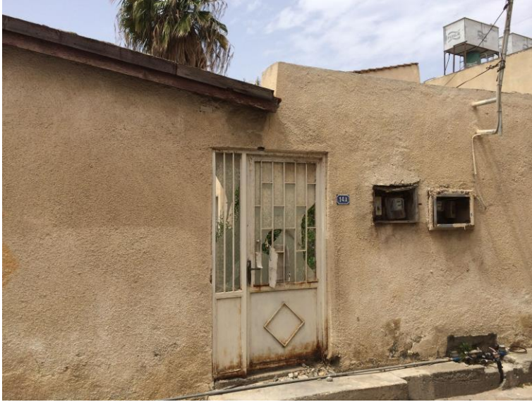
Figure 20. Bad Structural Condition (Street 3) Source: (Davoodi, 2014)
