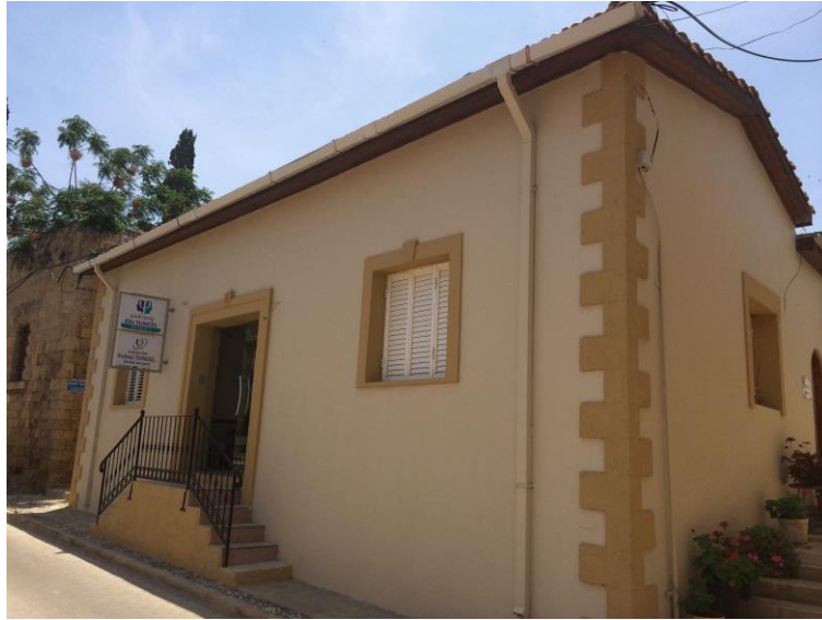
Figure 18. Very Good Structural Condition (Street 1), Source: Davoodi,2014)
