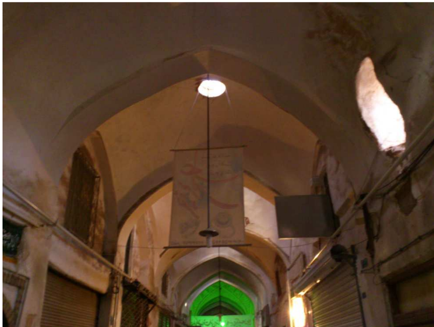
Figure 36: Roof opening in middle of roof in case number 3
