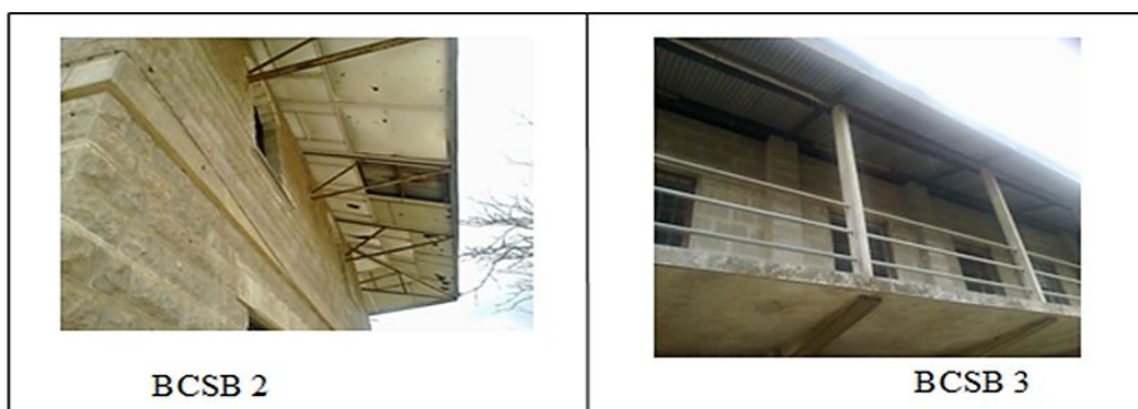
Figure 57: Steel and timber roof systems from Calabar cases (Hope Waddel Training Institution and Ederly Girls Secondary School)
