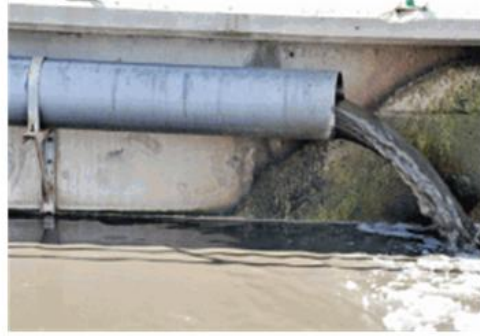
Waste water treatment in Bafra
