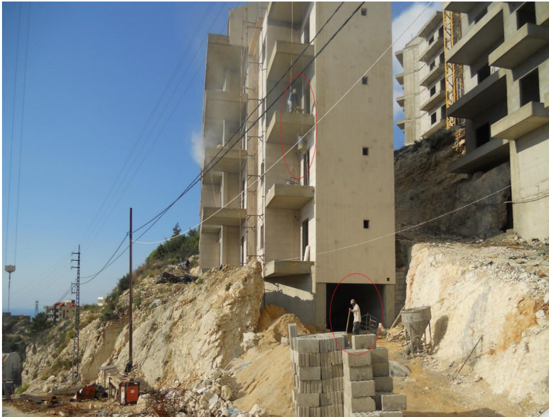
Figure 8. Worker at third floor is in danger of falling from height and the one at ground floor may be hit by a falling object.
