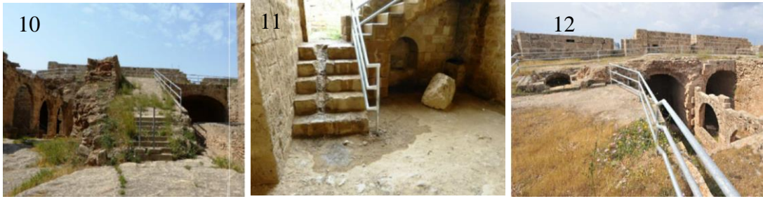
Figure 3.36: Different parts of upper level of Ravelin Bastion, (UNDP-PFF, Ravelin Bastion project, 2016).
