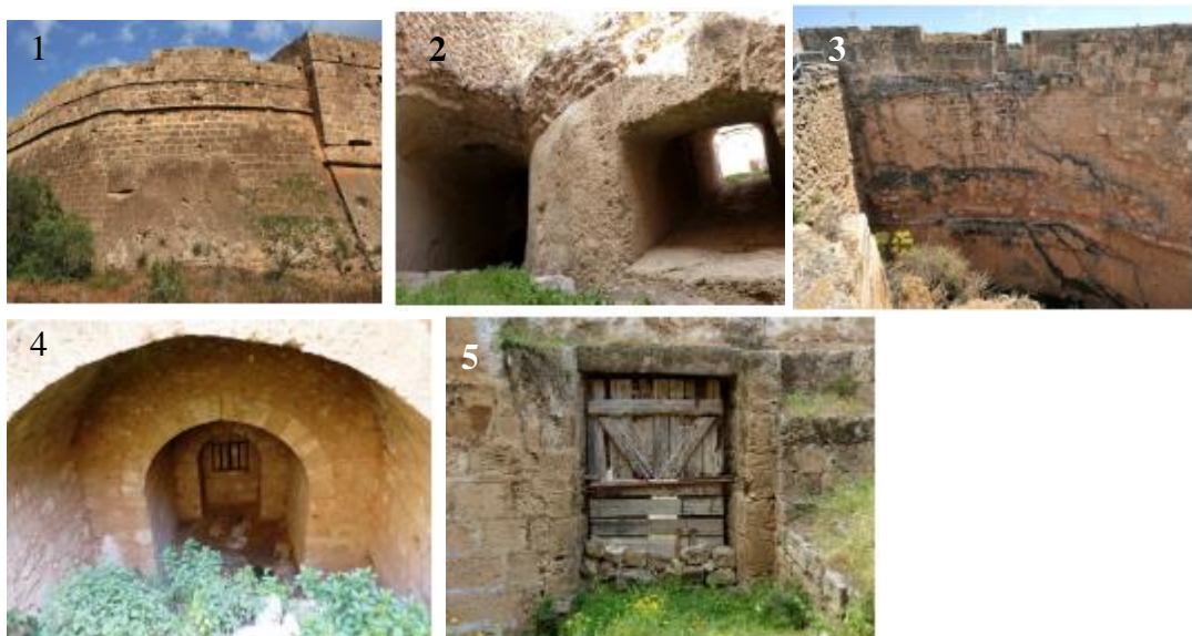
Figure 3.41: Different parts of lower level of Ravelin Bastion, (UNDP-PFF, Ravelin Bastion project, 2016).
