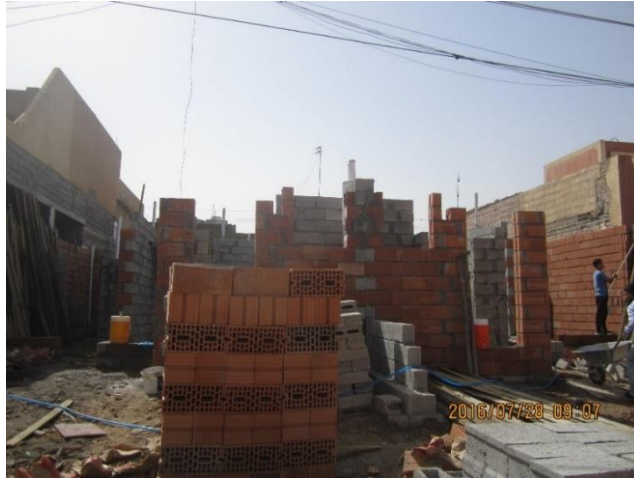
Figure 19: Poor Quality and Type of Materials Used for the Wall (Taken by author, 2016)
