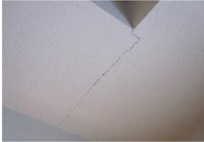
Figure 22: Cracks and Segregation at Roof Level (Taken by author, 2016)
