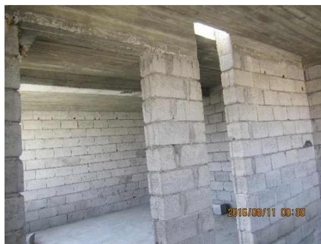
Figure 18: Lack of Thermal Insulation for the Wall (Taken by author, 2016)
