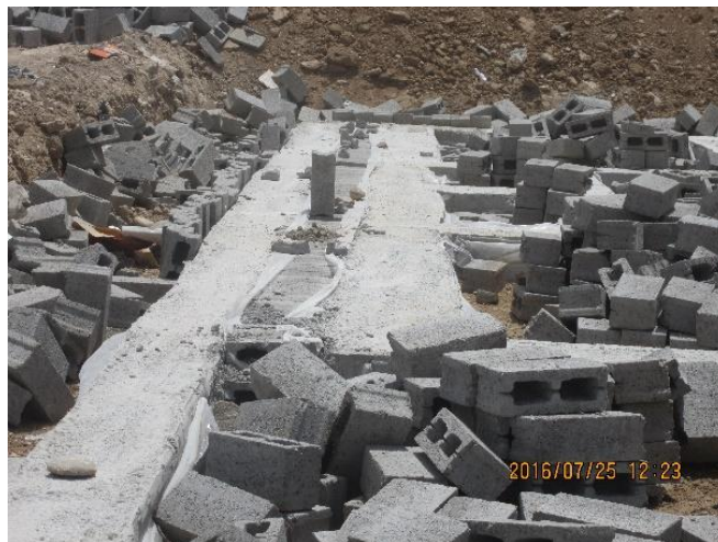
Figure 13: Lack of Foundation Design (Taken by author, 2016)
