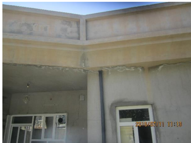
Figure 21: Lack of Waterproofing in the Roof (Taken by author, 2016)
