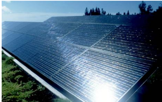
Figure 18: Photovoltaic solar panels [21]
