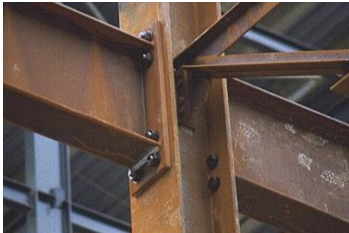
Figure 2.2: Truss Chord and gusset plates will be connected to the column web
