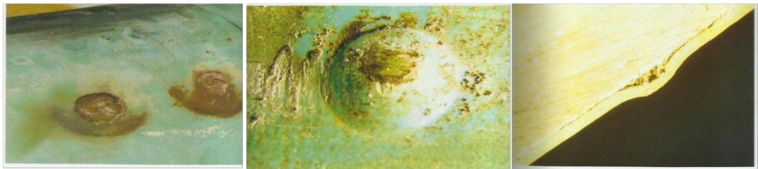
Figure 1.5: Corrosion under deposit [28]
