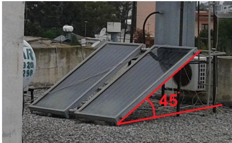
Figure 41. Tilted Angles of the Collector in Haci Ali Apartment in Famagusta
