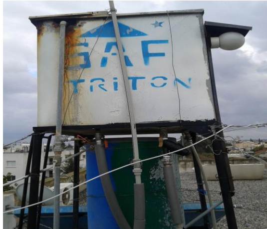
Figure 44. The insulation of Collectors in Haci Ali Apartment
