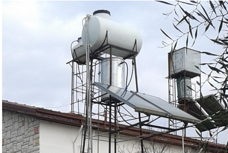
Figure 43. Height and Distance of Water Tanks of Solar Collectors in Social Housing Complex
