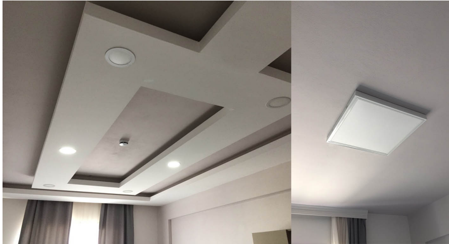
Figure 36: The LED lighting fixtures in Prime dormitory, (Photo taken by author).
