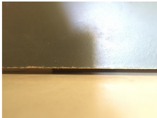
Figure 29: Air gap in the Kamacioğlu dormitory room doors. source : Author
