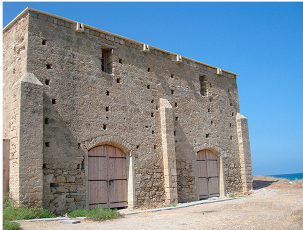
Figure 6. Small holes on the façade (Mersinlik 1) (Photo by Beser Oktay Vehbi).
