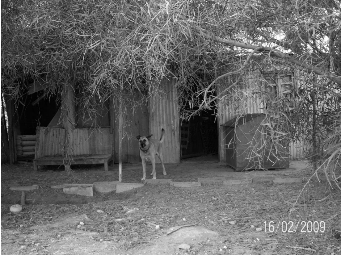
Figure 7. North facade of the steel shed, which has a timber structure and corrugated steel walls.
