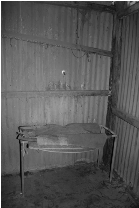
Figure 8. Remains of the kitchen sink in the steel shed.
