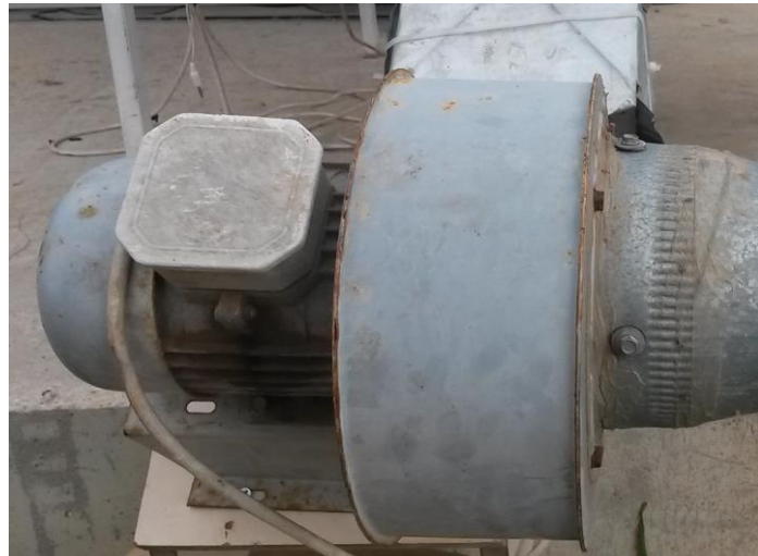
Figure 4.3: Photograph of collector Fan.
